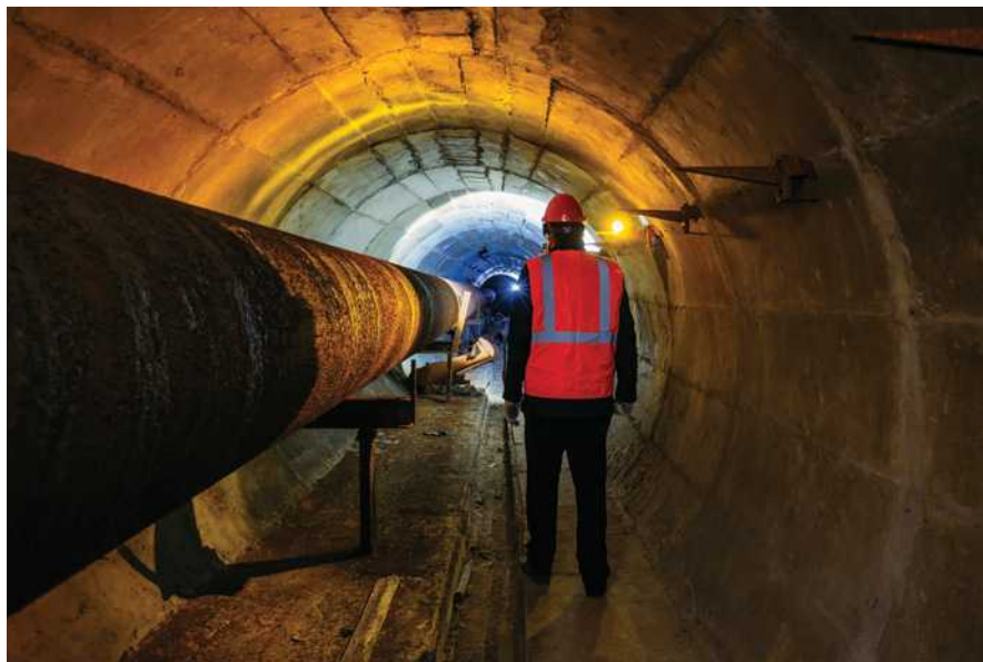
There are many overlooked spaces both inside and outside of health care facilities that can be classified as confined spaces.
