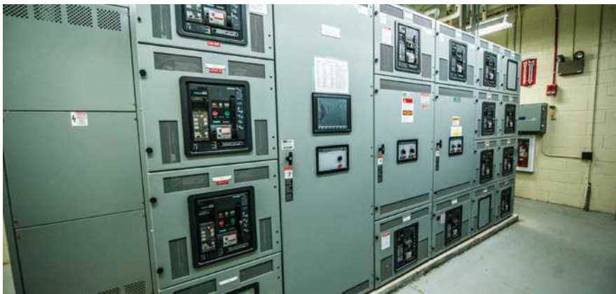
Synchronous gear for multiple generator sets is one of many items in the overall emergency power system to consider as a failure point.
