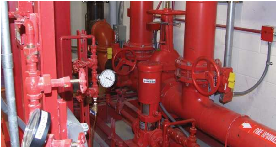
Fire sprinkler systems are dependent upon the public utility water source and delivery means.
